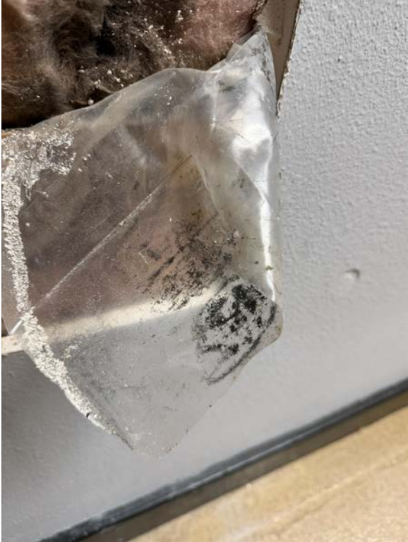
Visible Mold on Vapor Barrier
