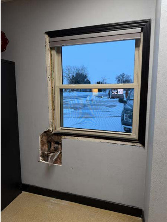
Exterior Wall of Day Room with Visible Mold
